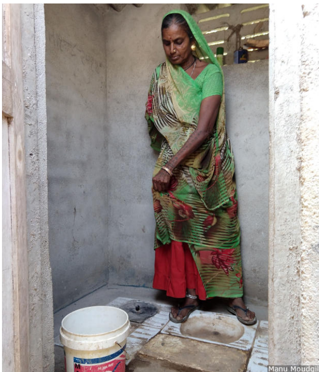
Dhari Ben explaining the functioning of the Ecosan toilet installed in her home in Gujada village of Gujarat's Bhavnagar district.
