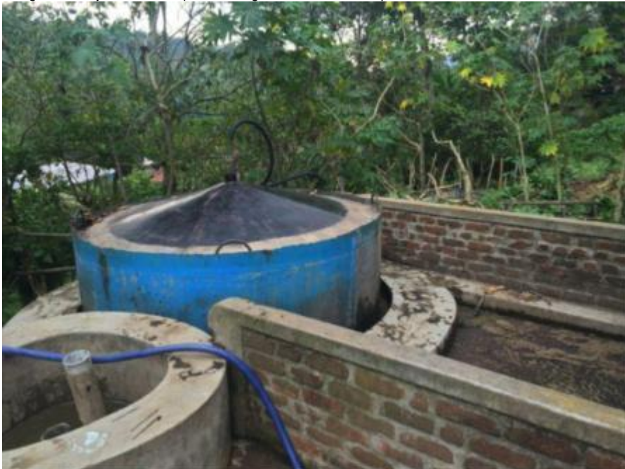
Here is one of the five Biogas plants at SHOLAI School
