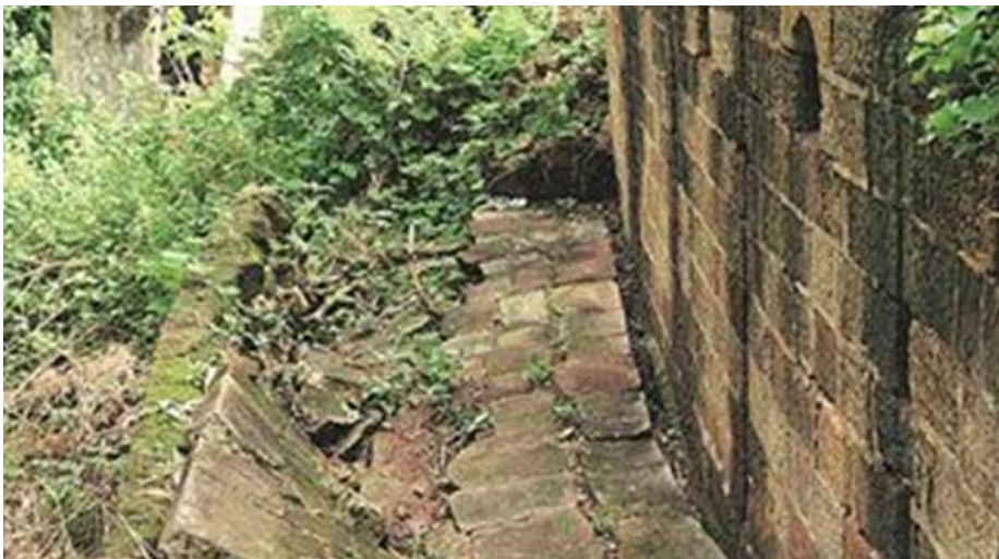
A corner of the fort that is yet to be cleaned Deepak Daware
